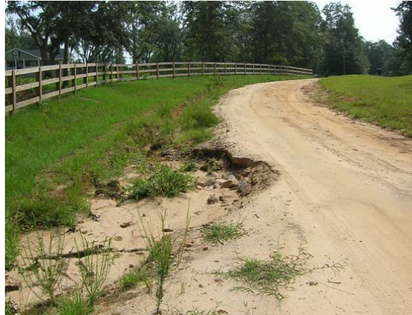
Ditch Failure Needs recrowning and drainage ditch installed
